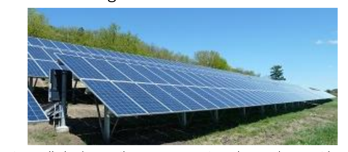
The River Falls (WI) 254-Kilowatt Community Solar Garden provides electricity to the community's renewable energy credit subscription program. A similarly sized solar project, or smaller, could offset the consumption of the Village government's energy use.
