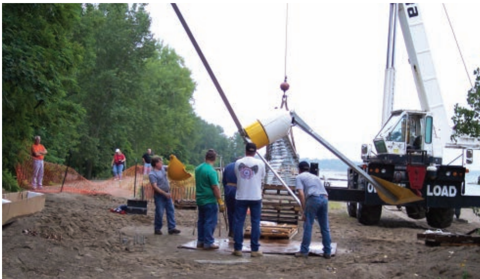
Volunteers help assemble and install Presque Isle State Park’s 10-kilowatt Bergey Excel wind turbine. The project was entirely paid for through a grant and donations of time, materials and money from local wind installers and individuals.
