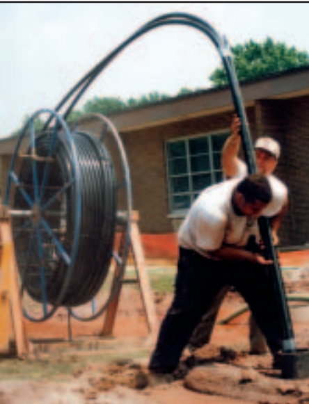
Photo: Advanced Energy
